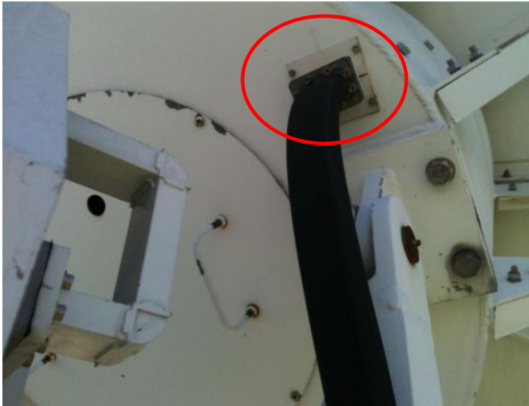
Figure 15 - View of the waveguide to be replaced
